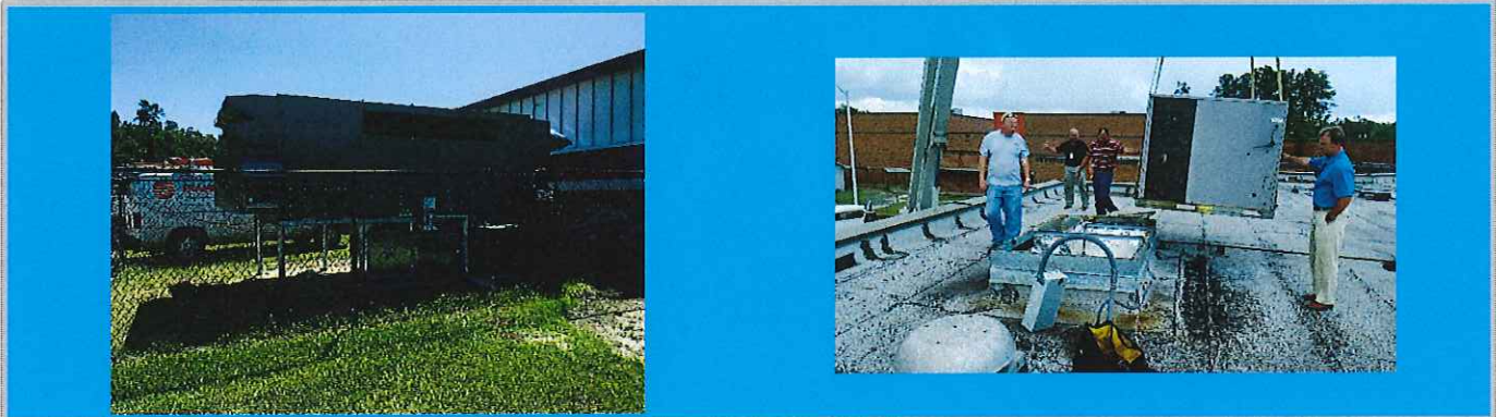
New Outside Air Unit @ Aynor Elem.
